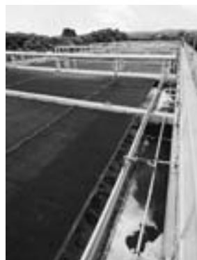
Wastewater treatment system
