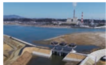
Construction of water gate of Nakata River in Fukushima [Kurehanishiki Construction Co.]
