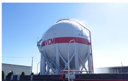
Sprinkling water on high-pressure gas tanks
