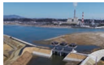
Construction of water gate of Nakata River in Fukushima [Kurehanishiki Construction Co.]
